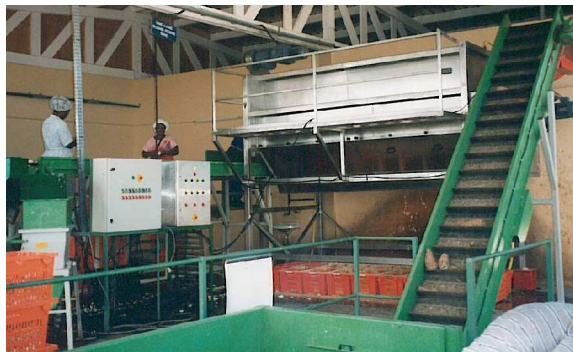
Overall view with storage bin and feeding belt (in front), DORNOW Peeling Machine (at the back) and inspection belt for peeled products (at the back, to the left).
